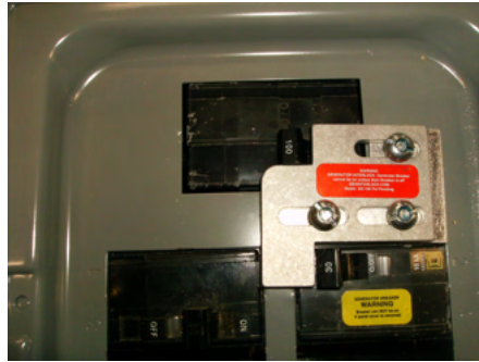
QO Generator On
