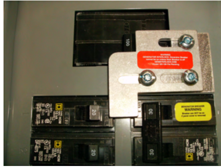
Homeline Generator on
